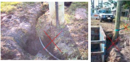
Above: Poles with become unstable if undermined
